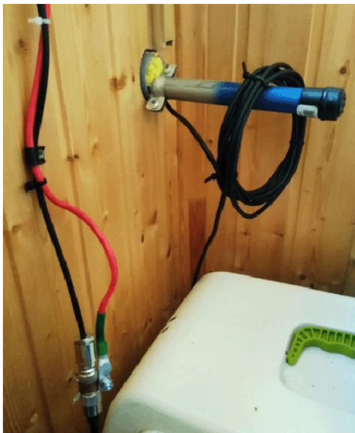
Figure 4 Round Counterpoise Inside of Balcony
