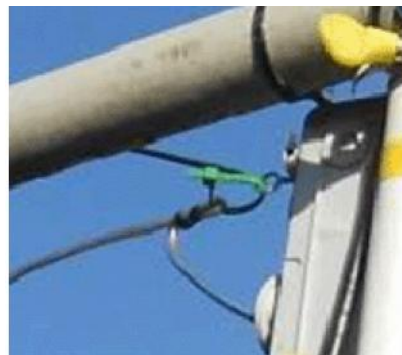
Picture 5 Horizontal Wires at Connection Box
