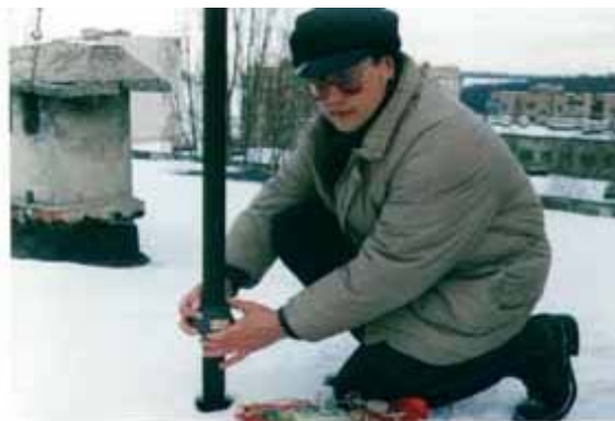
Photo: Ferrite core installed at the antenna mast base
